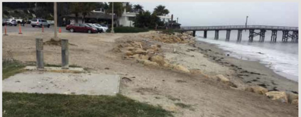
The GSD Vault (lower left square metal top), houses the infrastructure connecting wastewater plant and ocean outfall. It sits at the edge of Goleta Beach, which is eroding rapidly. (Hillary Hauser photo)
